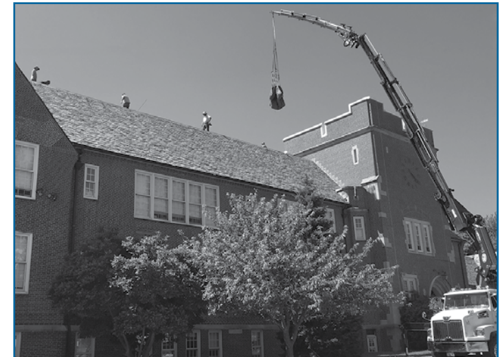
The district completed the first phase of the project (new and repaired roofs) last summer at nearly $1.2 million under budget.
